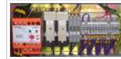
Power House Monitors power management
